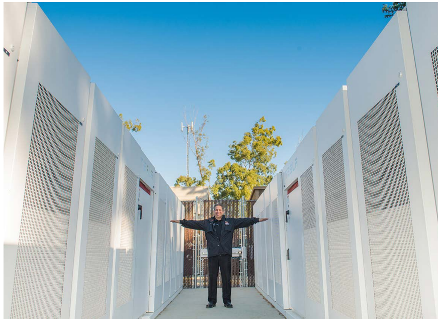
Kenny Seeton, central plant/energy manager at CSUDH, stands among 20 Tesla battery banks. Photo credit: CSUDH Office of Communications
