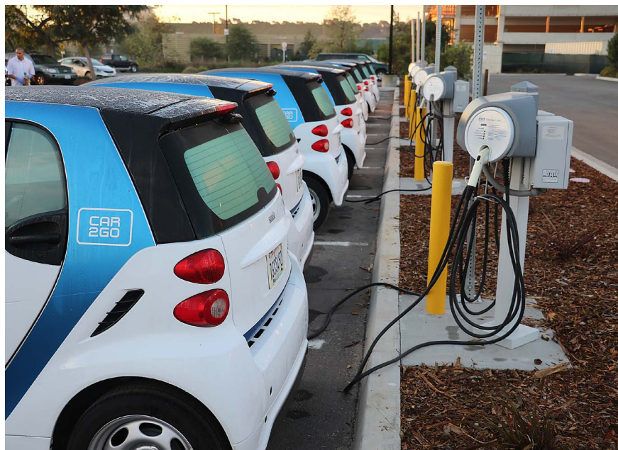
University of California, San Diego leading in EV charging and affordability. Photo credit: Rhett Miller
