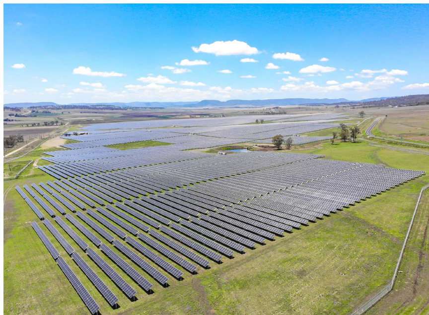
University of Queensland's 64 MW Warwick Solar Farm powers UQ to be 100% renewable. Photo credit: Sarah Haskmann
